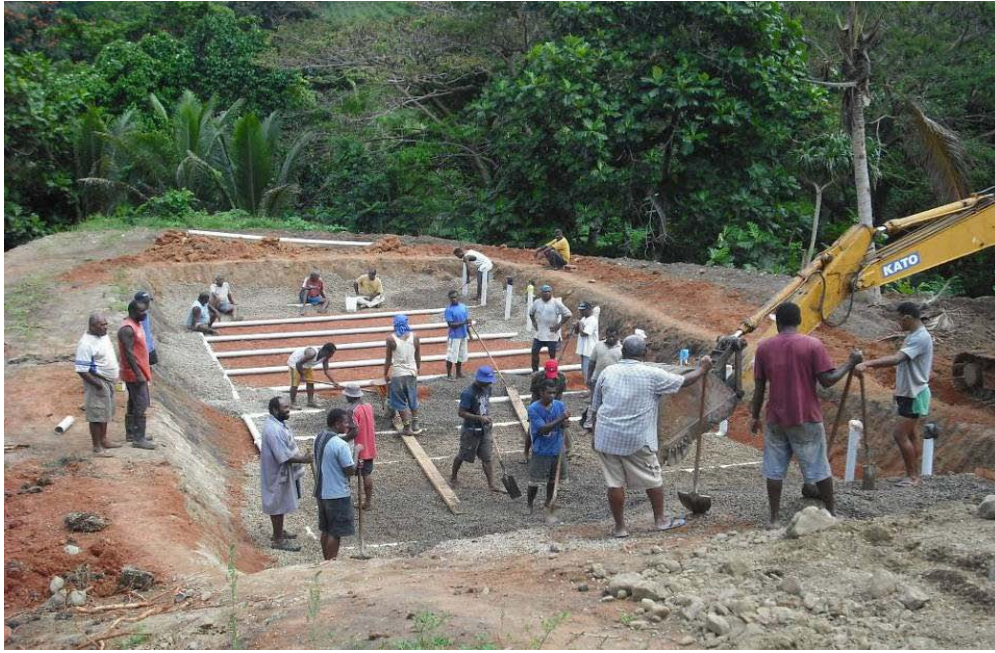
Fig. 1: Villagers constructing a vertical-flow wetland as the first stage of a village-scale black-water treatment system, Votua, Fiji.
